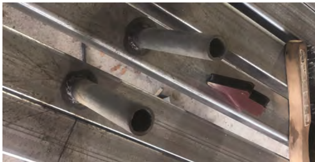
Figure 4: 6" nipples are attached every four feet along the length of both skids. Each side includes seven nipples. These nipples will receive the top rail hoops.
