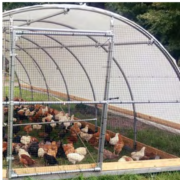
Figure 5: Two of three purlins can be seen in this photo on the inside of the hoops along the ridge and the right side. A third purlin is attached to the other side of the hoop.
